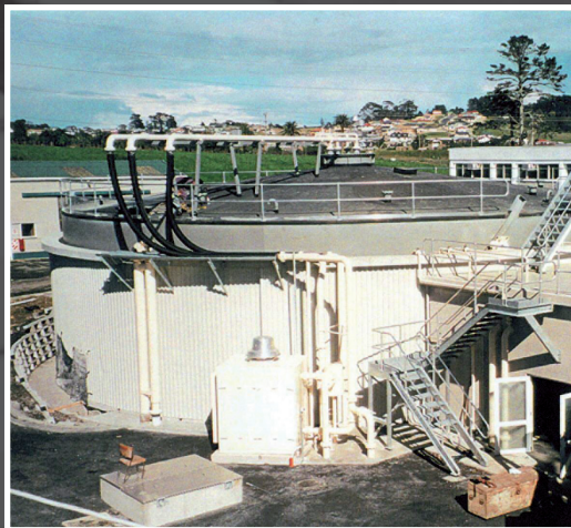
North Shore WWTP upgrade Balance of plant contract North Shore City Council
